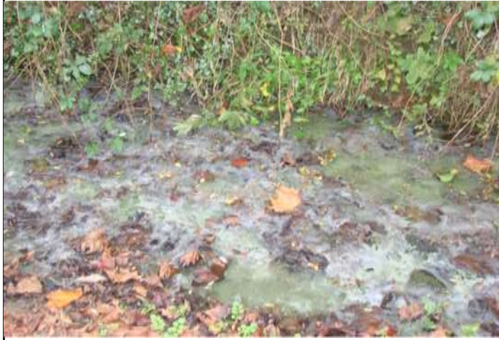
DWWTS - Septic tank
